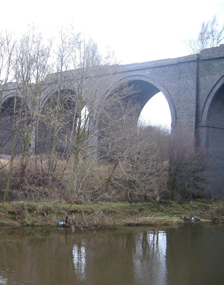
Bradley Viaduct showing loss of parapet
